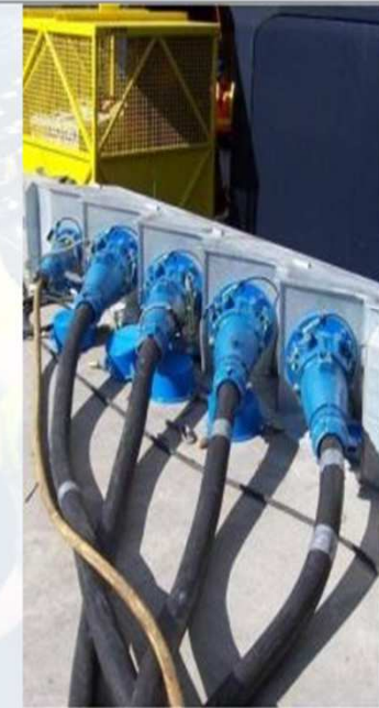
The cables plugged into the power outlet
